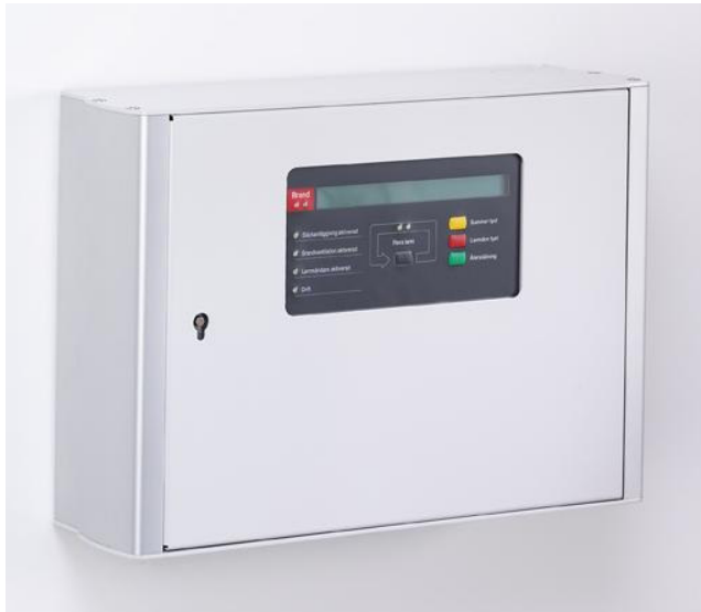
Figure 1. The external Fire Brigade Panel 1826 with the 2 nd generation of the cabinet.
